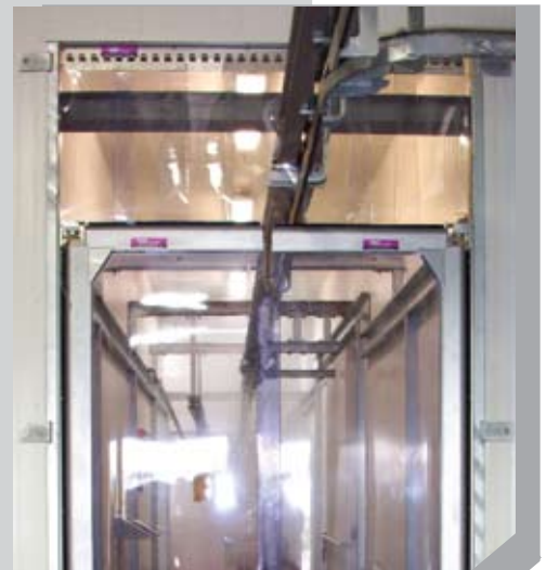
Double PVC swing door and strip door sealing to the meat rail
