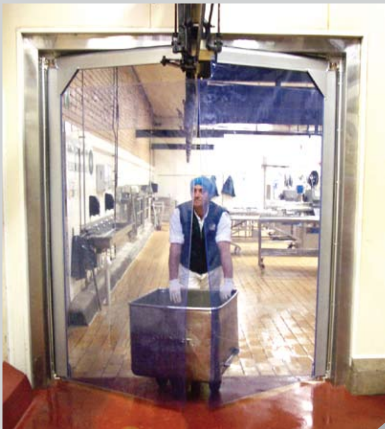
Enhances hygiene, isolates critical functions, prevents cold air loss and stabilises the temperature
