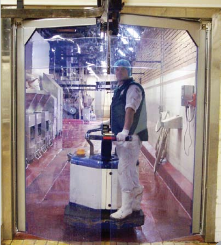
PVC swing door allows convenient access for personnel, trolleys and conveyancing equipment
